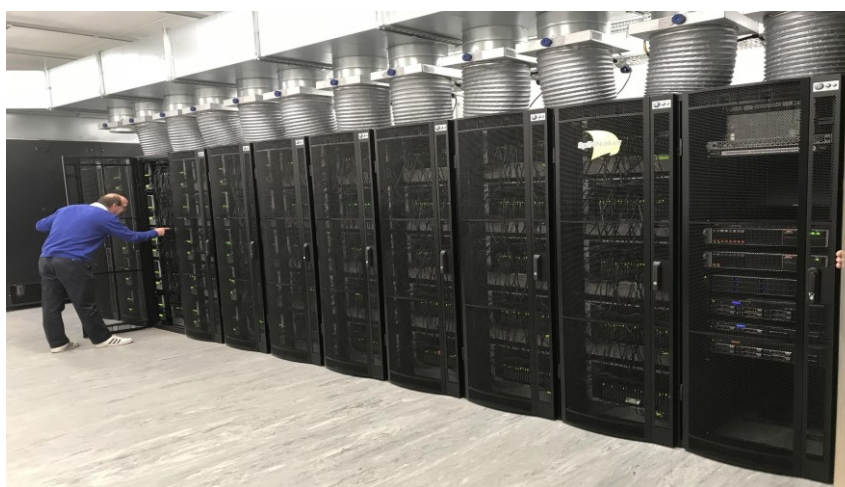
Figure 1. The million-processor SpiNNaker machine at the University of Manchester
